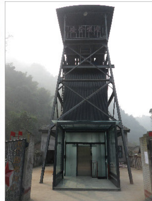
黄村井井下电梯 Huang Cun Jing Under-Well Elevator
